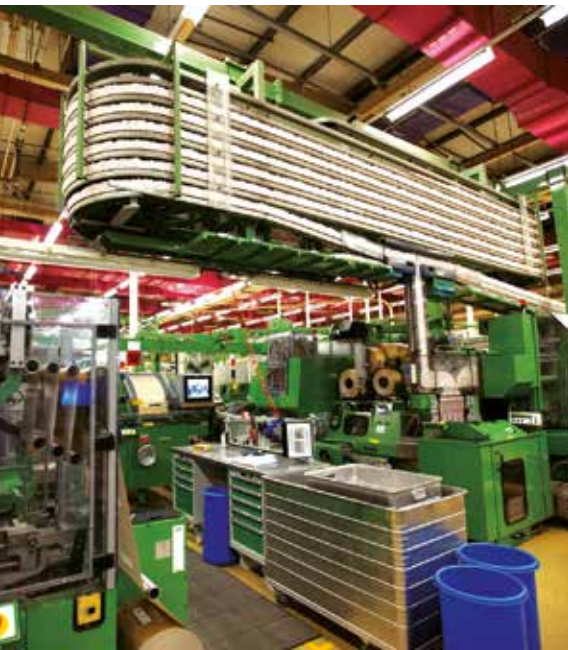
UHS packing line within new extension
