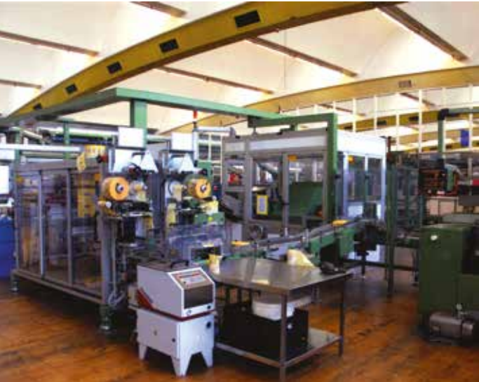
New high-speed line installed in South factory
